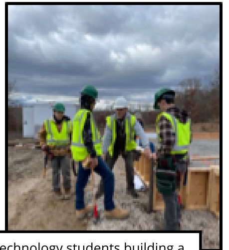
CHARIHOTech Construction Technology students building a home in Hopkinton with South County Habitat for Humanity
